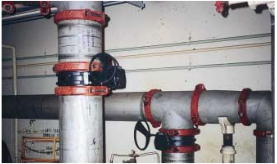
A complete system of stainless steel products is ideal for deionized water, chemical and related systems.
