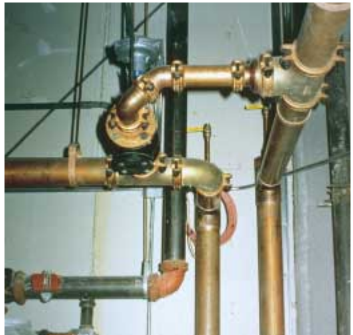
The copper connection for plumbing services.
