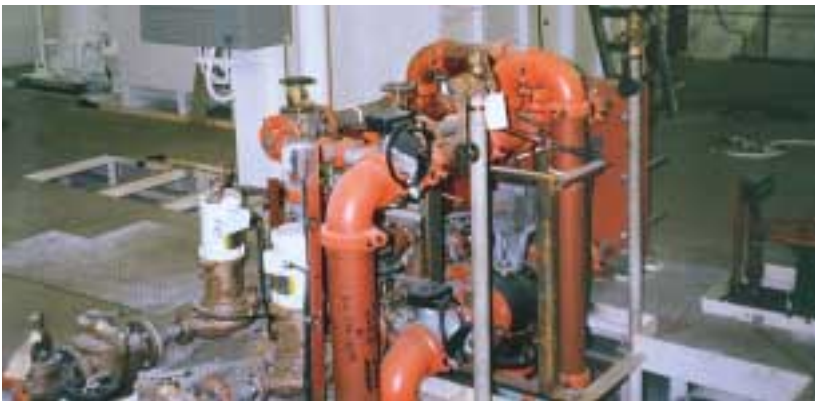
Marine shipboard piping utilizes rigid and flexible couplings to accommodate special needs.
