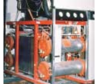
Heating, cooling and plumbing equipment.
